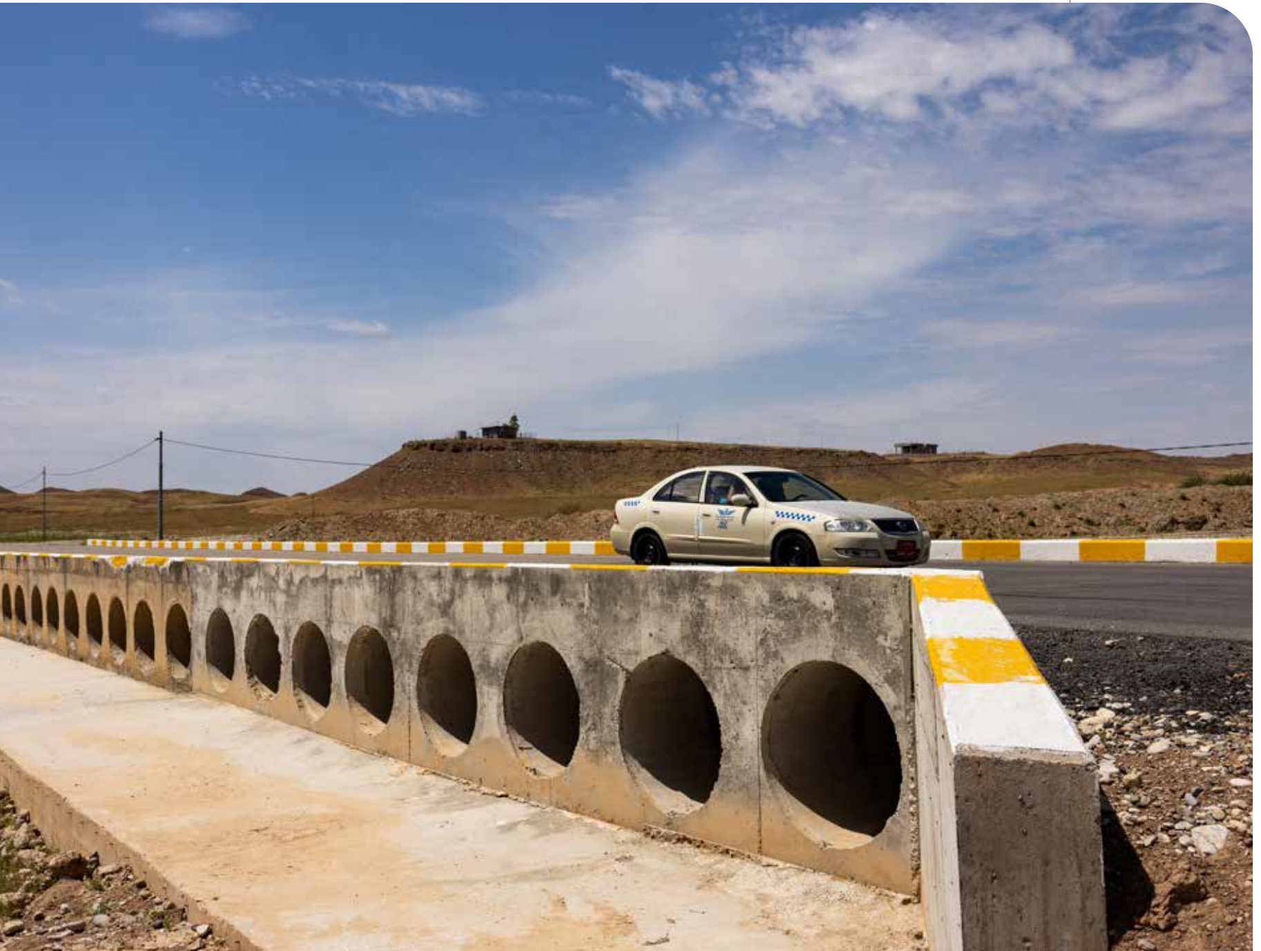
After torrential rains washed away the major bridge to Qadir Karam, Pearl Petroleum rebuilt the major artery, which connects the surrounding villages
